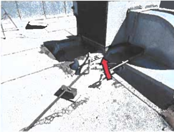
Photo #3 RTUs are not provided with seismic restrains.
