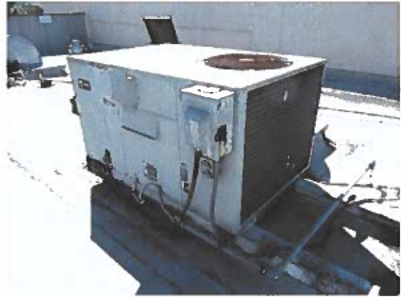
Photo #2 Side view of typical 3-ton RTU.
