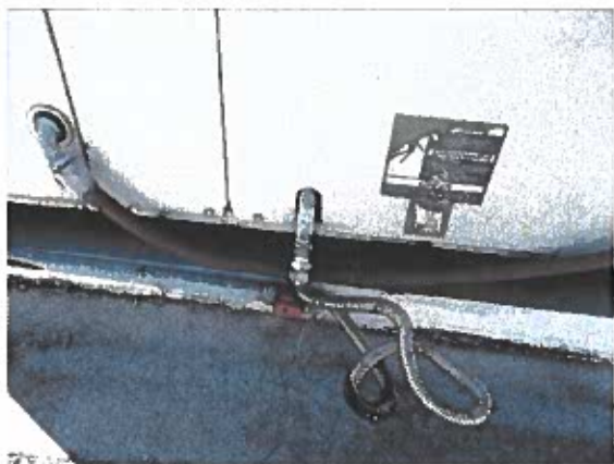
Photo #5 Typical natural gas pipe routing to the RTUs.
