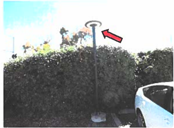
Photo #34 Typical external pole lighting fixture.
