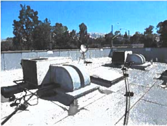
Photo #1 View of two 3-ton RTUs on the lower level roof.
