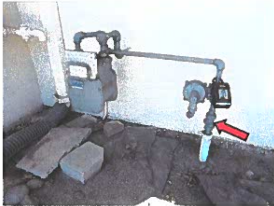
Photo #35 View shows natural gas meter, seismic shutoff valve is not provided per code.
