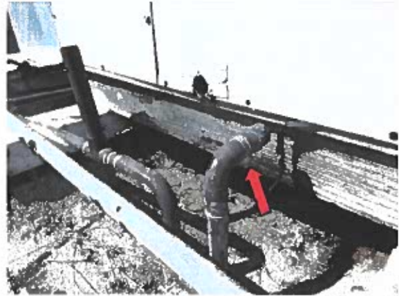
Photo #4 View of broken condensate water drain pipe.
