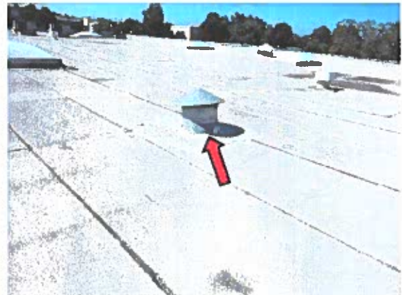
Photo #10 Typical air vent located on upper roof level
