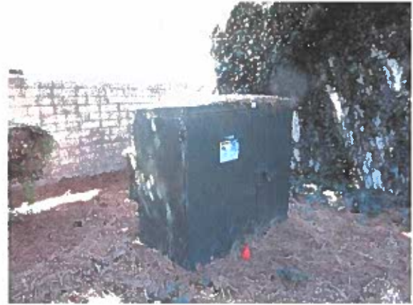
Photo #14 View of the pad-mounted, utility-owned transformer located in the back side of the building.
