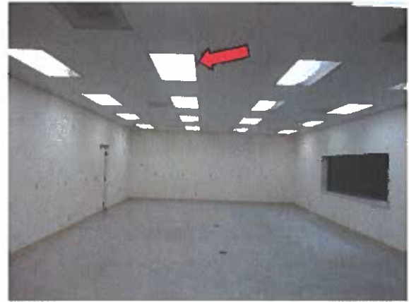
Photo #16 Typical T-8 fluorescent lights in the additional room to offices.
