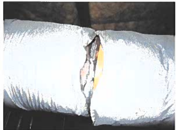
Photo #29 View shows damage in the duct insulation.
