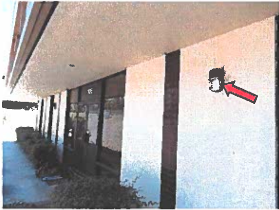
Photo #32 Typical external lighting fixtures needs to be cleaned and maintained.
