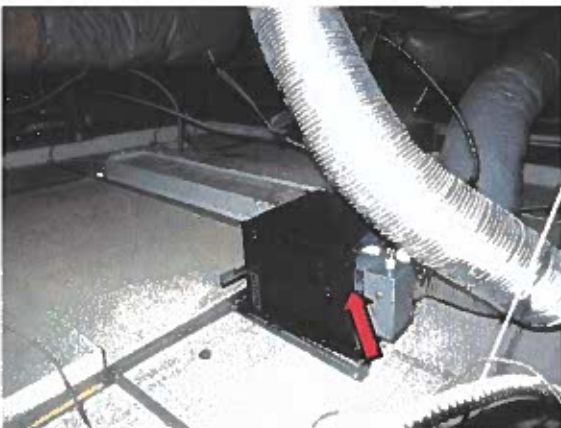
Photo #30 View of the exhaust fan above the ceiling provided to the break room.
