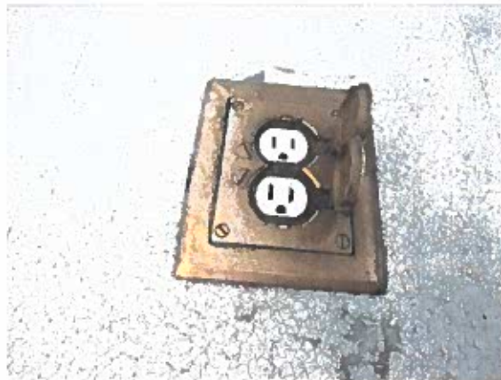
Photo #17 Typical floor mounted electrical power receptacle switch in the additional room
