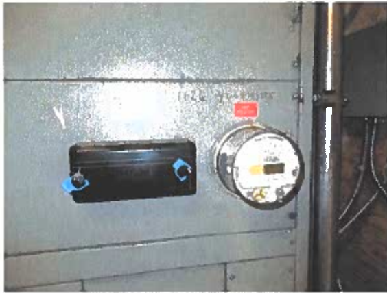
Photo #13 View of the main electrical meter.
