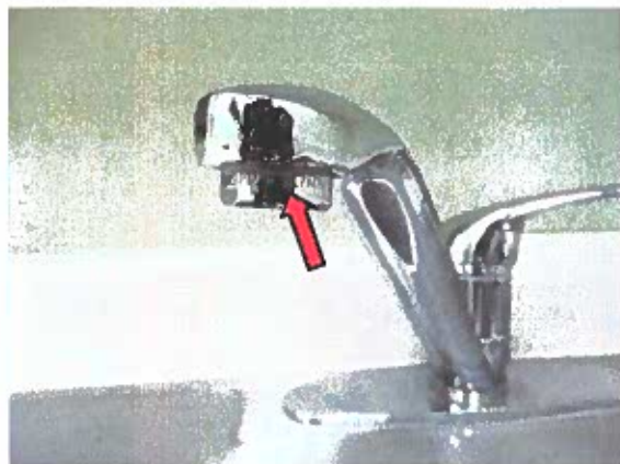
Photo #23 Typical view of water-efficient faucet provided in the break room sink.
