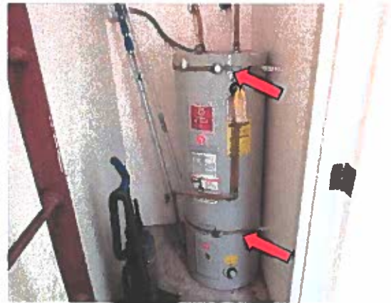
Photo #20 View of 50-gal. electric water heater located inside janitor room and provided with seismic restraints.
