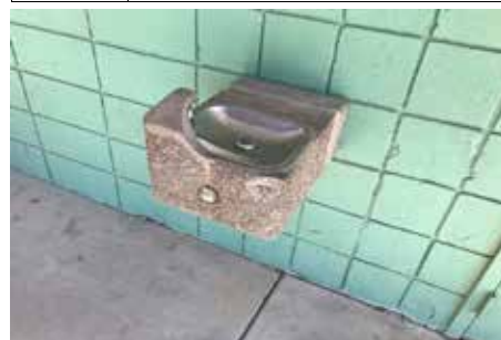
#24 AUGUSTINE DRINKING FOUNTAIN, DAMAGED
