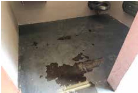
#62 PINEWOOD EPOXY FLOOR COATING DEGRADATION
