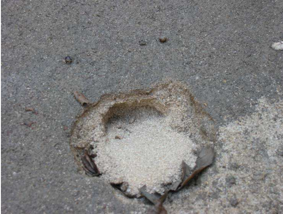
Figure 7 Formation of Clogging Crust on Filter Bed
