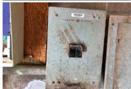
#72 SINNOTT DISTRIBUTION PANEL
