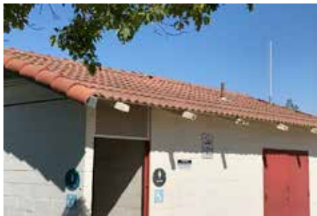
#29 GILL, DAMAGED RAFTER TAILS
