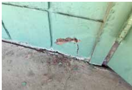
#21 DETERIORATION AT AUGUSTINE
