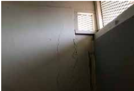
#65 FOOTHILL PARK, STRUCTURAL CRACK
