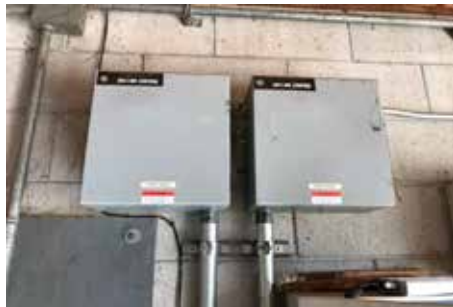
#31 GILL, LIGHT DIMMING PANELS
