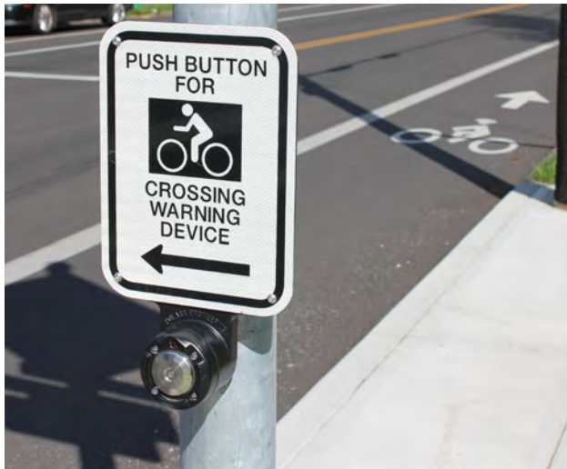
User-activated button mounted on a pole
