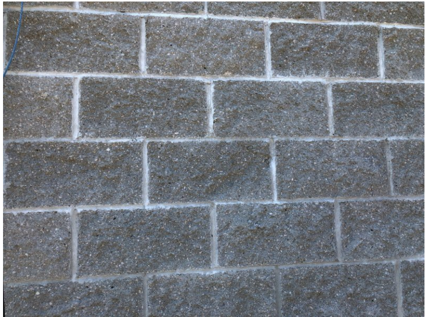
Cracks, back side
