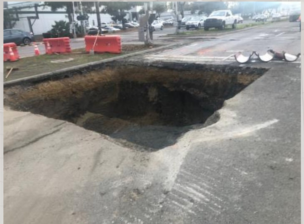
Sink hole at Montague Expwy., Milpitas (January 11, 2019)
