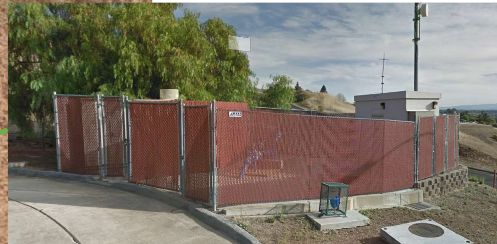
Hillside Pump Station aka – Country Club Booster Pump Station
