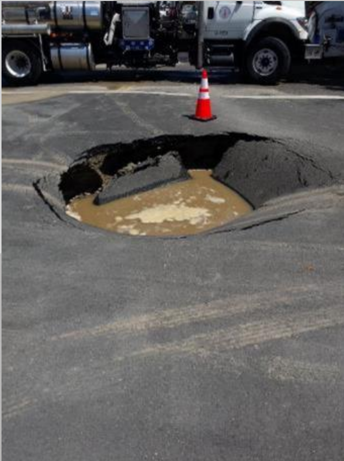
Sink hole at Technology Drive, Milpitas (January 6, 2019)
