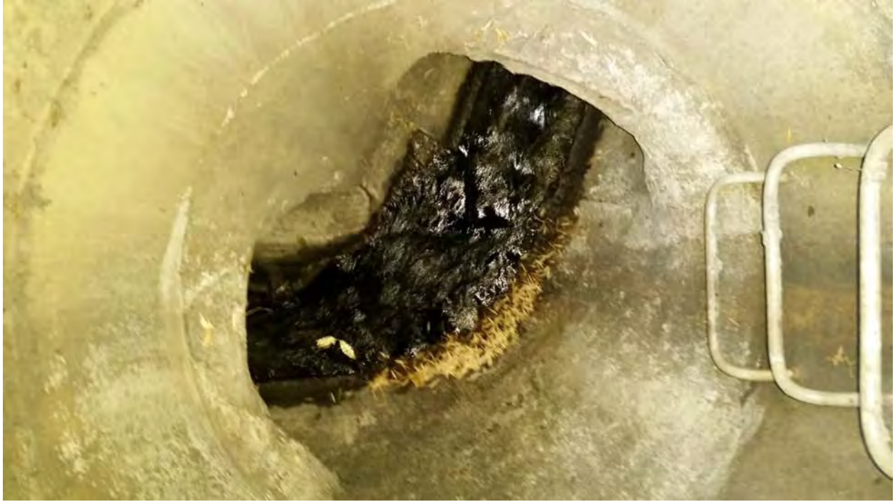
Storm Water Receptacle, SW3
