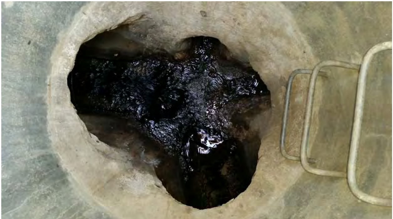
Storm Water Receptacle, SW2
