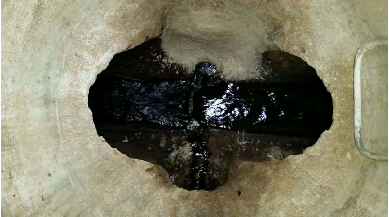
Storm Water Receptacle, SW1
