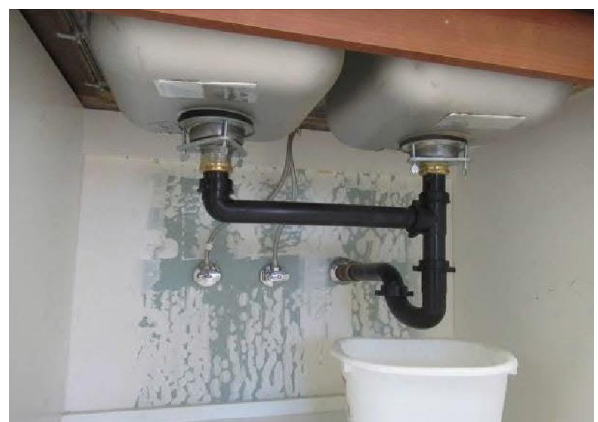
Photo #24 Typical view of sanitary drainage PVC pipe.
