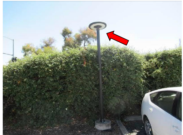
Photo #34 Typical external pole lighting fixture.
