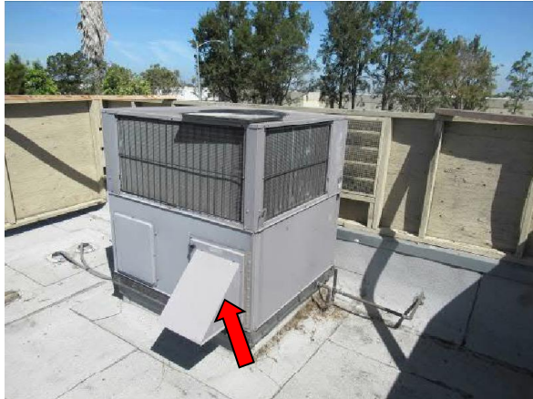
Photo #7 View of 4-ton DX RTU with adjustable outside air intake.
