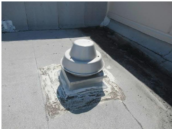
Photo #9 View of the restroom exhaust fan located on the lower roof level.
