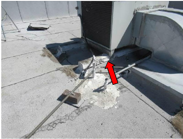
Photo #3 RTUs are not provided with seismic restraints.
