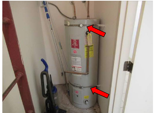
Photo #20 View of 50-gal. electric water heater located inside janitor room and provided with seismic restraints.
