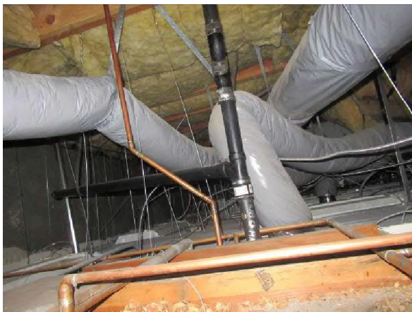
Photo #28 Typical view of above ceiling shows some of the plumbing piping and flexible ducts.
