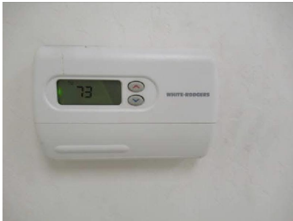
Photo #19 Typical wall mounted electronic thermostat.
