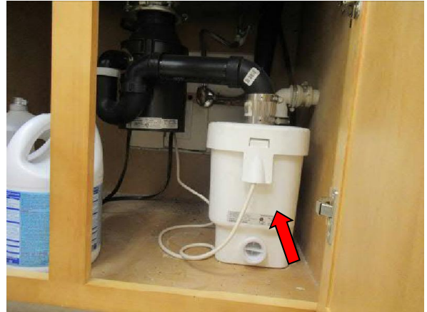
Photo #27 View shows the industrial sink drainage collected and pumped to the sink in the janitor room with water pump.
