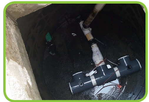
Manifold Tee View of a Cleaned System
