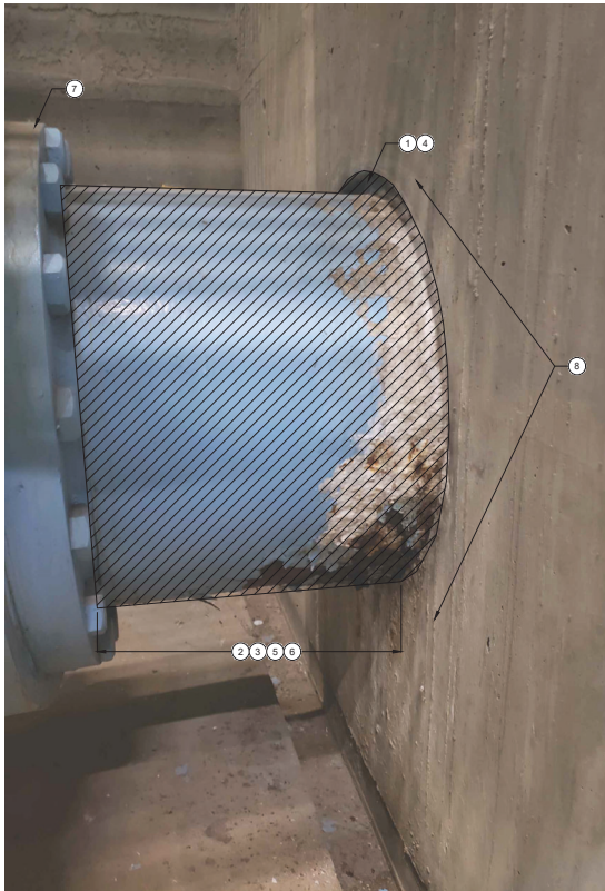
PHOTO 1 - PUMP NO. 5, 6, 7 18" SUCTION PIPING TO BE REPAIRED
