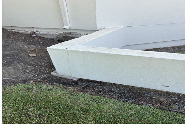
TYPICAL STUCCO CRACKING
