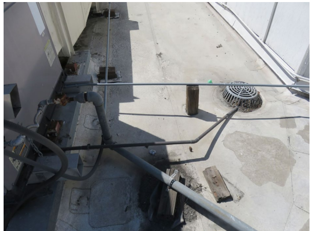
Gas piping, condensate drain, and roof drain near AC-2
