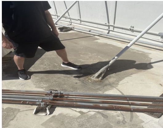
AREA OF FAILED ROOF DECK AND ROOFING
