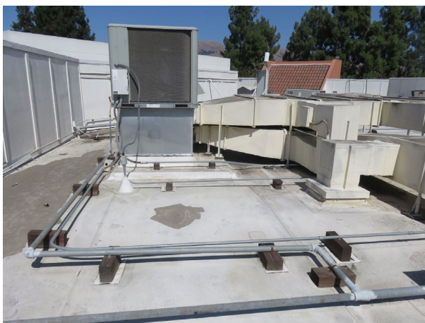
Gas piping near AC-3
