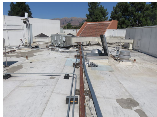
Gas piping near AC-4
