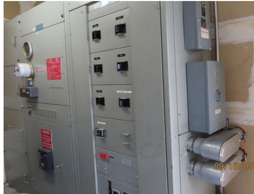
MAIN DISTRIBUTION SWITCHBOARD "MSB2"
